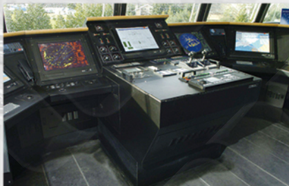
航海设备 Navigation equipment
